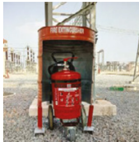
▲ Canopy Arrangement for Fire Extinguisher
