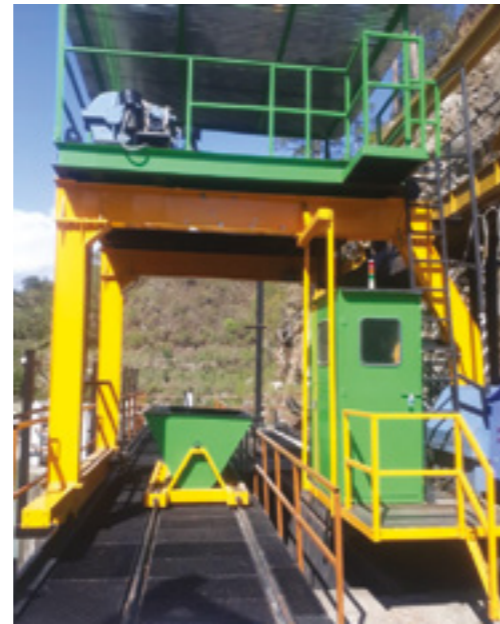
▲ Trash Rack Cleaning Machine at Swasti Power Private Limited
