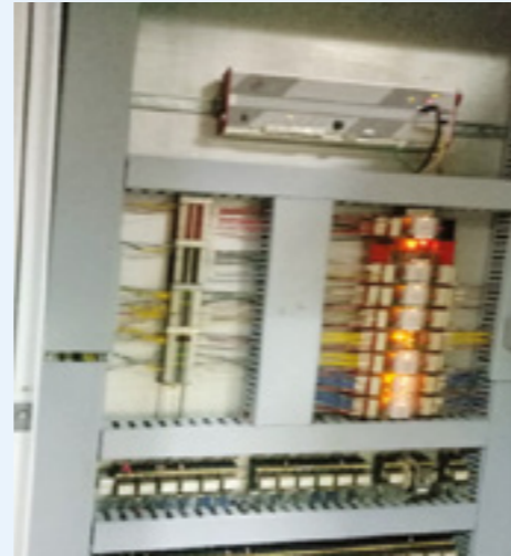
▲ Modified PLC at Bhilangana Hydro Power plant
